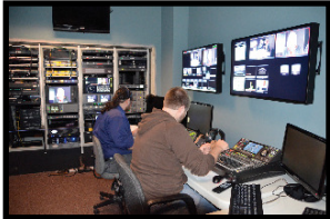
New Master Control Room
